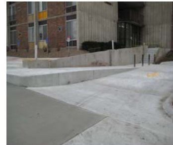
New drop off area in front of JI to be finished in 2010
